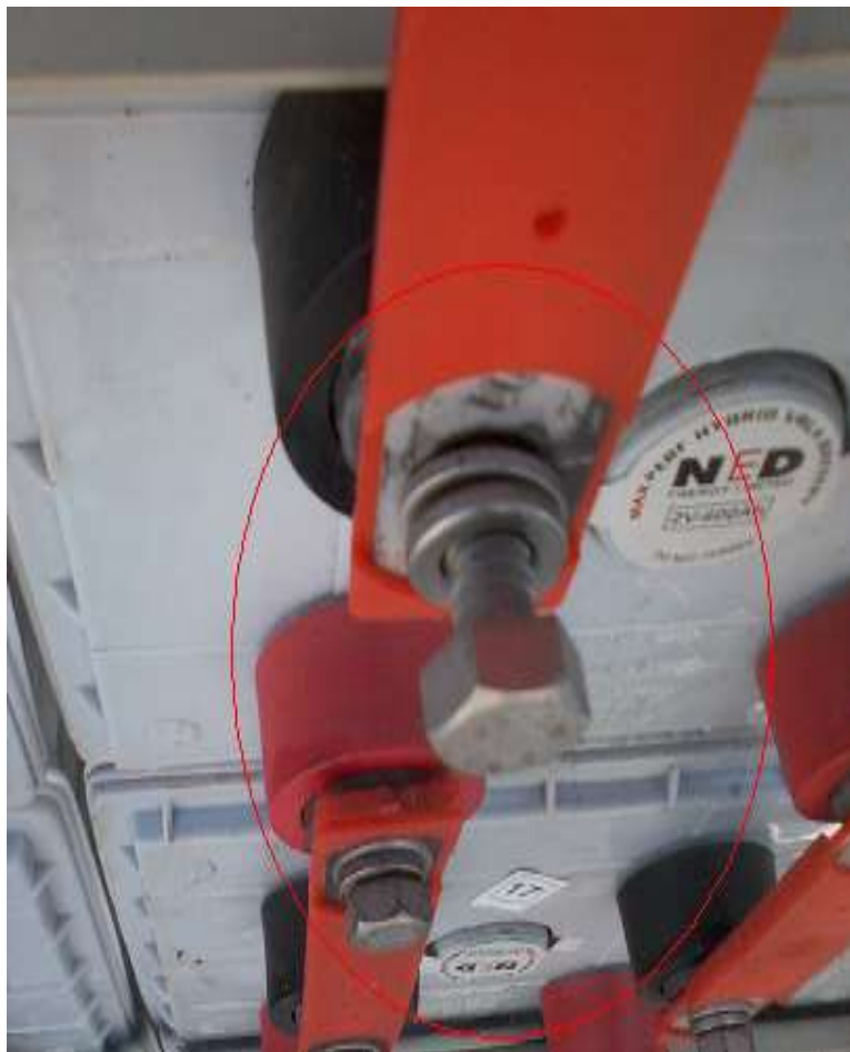
Battery Bank terminals tightening not done
