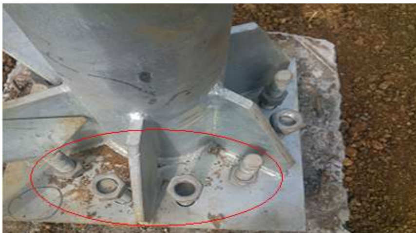
TIGHTENING NOT DONE
