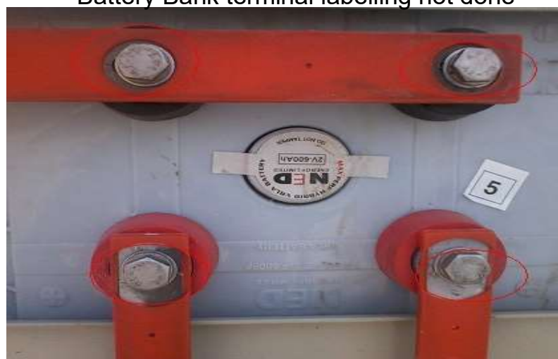
Battery Bank terminals safety caps missing and BB cell serial number is not available
