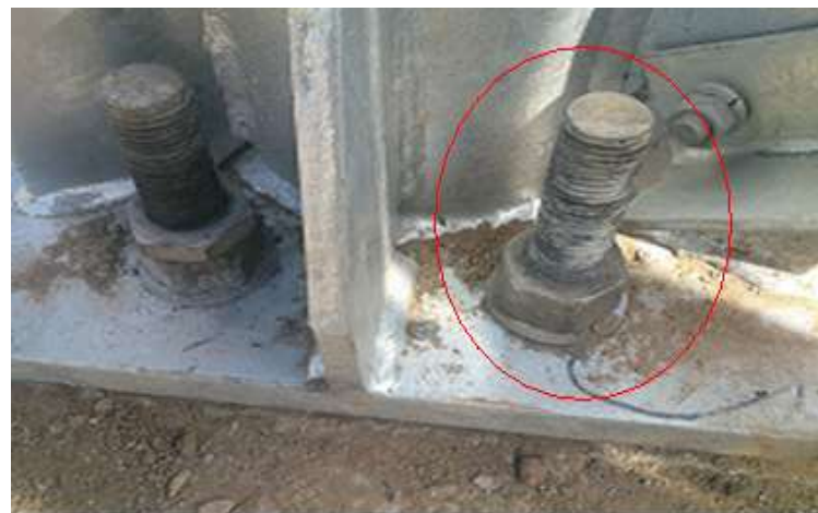
LOCK NUTS MISSING
