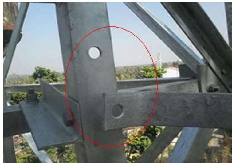
NUT BOLT MISSING
