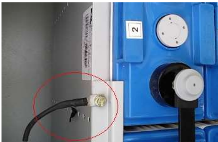
BB earthing cable color code not maintained
