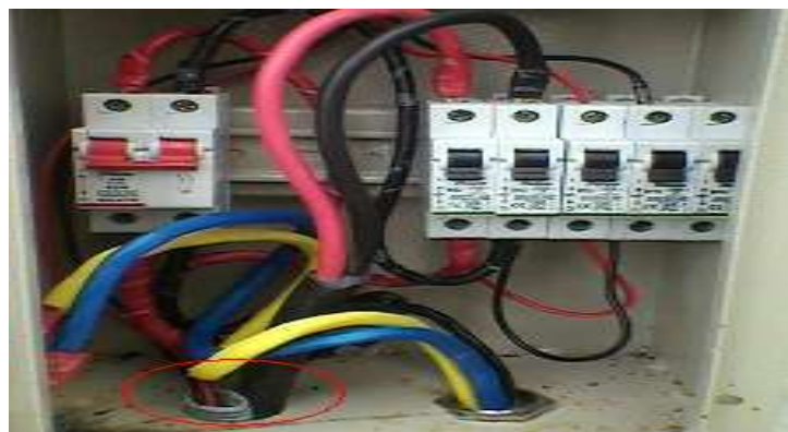
M Seal not provided for cable entry points
