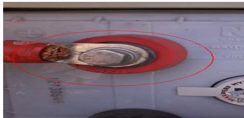
Battery Bank terminal labelling not done
