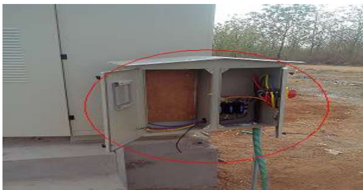
EB Meter box cables not connected
